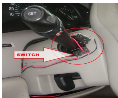
Fig. 9 Part of the LDW system showing the two switches connected with the turn signal control.
