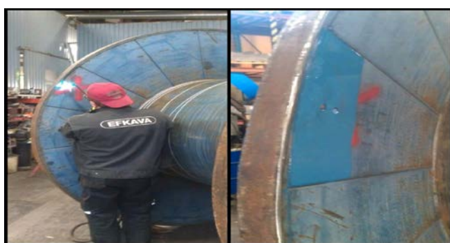
Figure 19: Example of drum damage reparation
