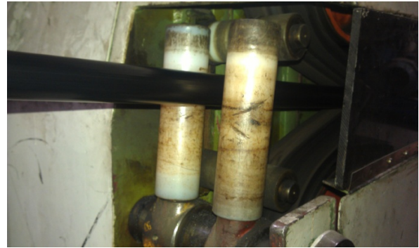
Figure 16: Example of damaged rollers
