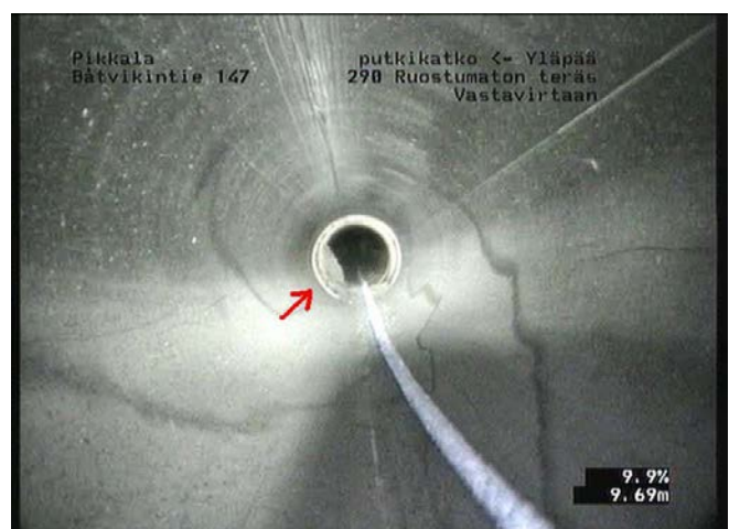
Figure 17: By-product mass in the CCV curing pipe
