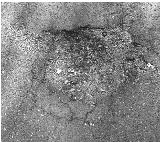
Figure 3: Picture of the overdriven pothole to measure the sound pressure level.
