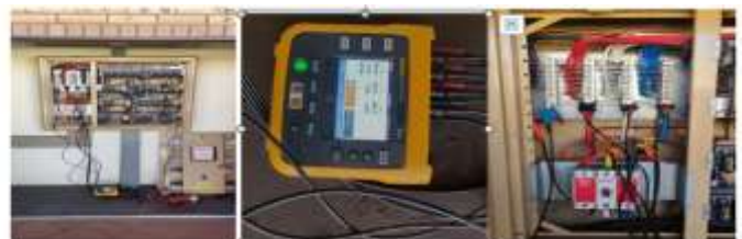
Fig. 8: Fluke 1738 Three-Phase Power Logging Process
