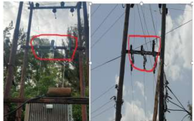
Fig. 11: Some of Unprotected DTs against Lightning
