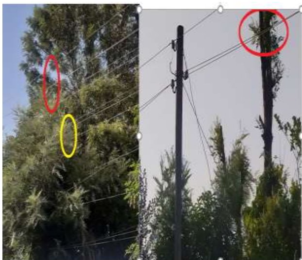
Fig. 12: MV and LV lines are in Contact with Tree Branches
