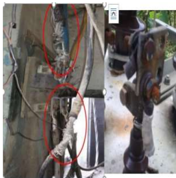
Fig. 13: Damaged DTs part due to poor cable termination
