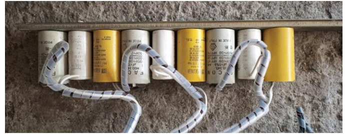
Fig.13: The array of capacitors
