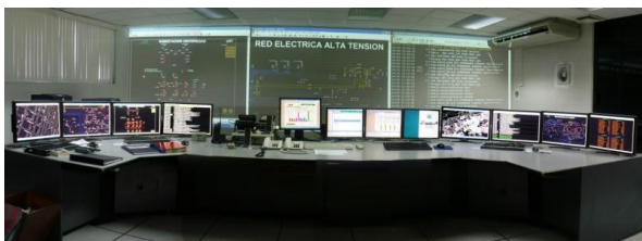
Fig. 1. Typical view of a Distribution Control Center.
