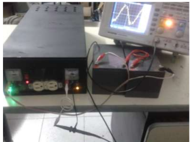
Fig. 19. Inverter operating with the photovoltaic system.
