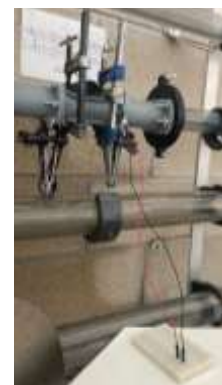
Fig. 15: Motor connection to the board
