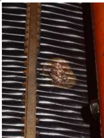
Fig. 2. Internal short-circuit of 167 MVA/500/220 kV autotransformer regulating windings.
