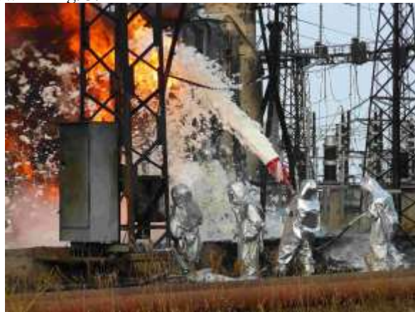
Fig. 3. The emergency at the 500 kV electrical substation with damage and fire of a three-phase autotransformer group.
