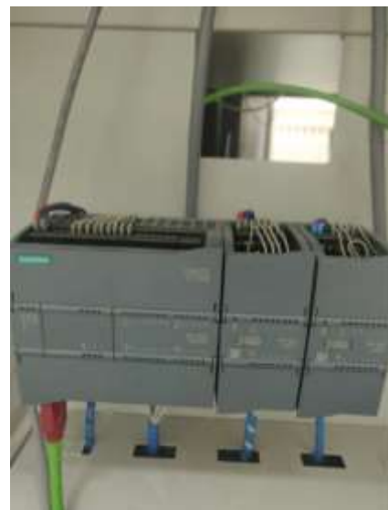
Fig. 7: Logical and control block with PLC of digital twin stand
