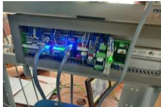
Fig. 6: Terminal block of digital twin stand
