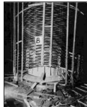
Fig. 5: Photo of phase “B” of the low voltage winding of 250 MVA / 220 kV transformer, illustrating the loss of the axial stability of the winding, i.e. the movement of the winding in the axial (vertical) direction under the action of electrodynamic forces during the flow of short-circuit currents
