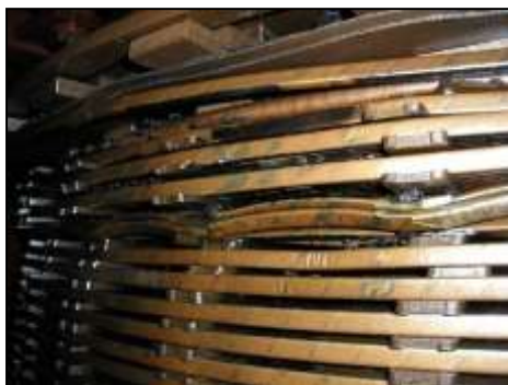
Fig. 8: Residual deformations of the HV winding of 250 MVA/500 kV/110 kV autotransformer with twisting of the winding and lodging of the turns on the edge
