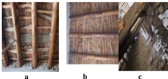
Fig. 3: Damage by termites to flooring materials made from Populus (a,c) Salix (b) trees
