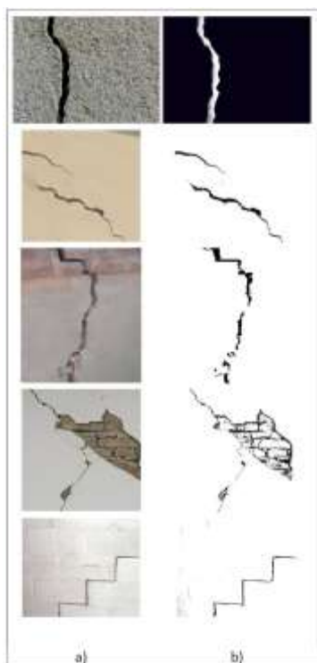
Fig. 10: Classification of the different types of cracks detected.
