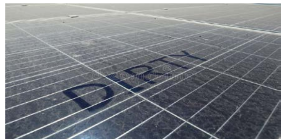
Fig. 2: Dust of solar panels
