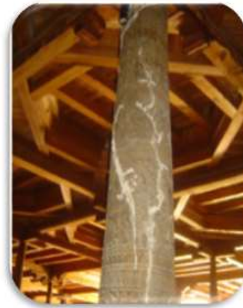
Fig. 7: Termite tunnels in wooden columns
