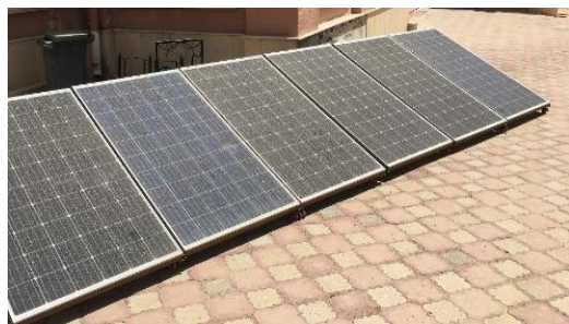
Figure 3: Tested solar panels held on 30° tilted holders facing South direction.
