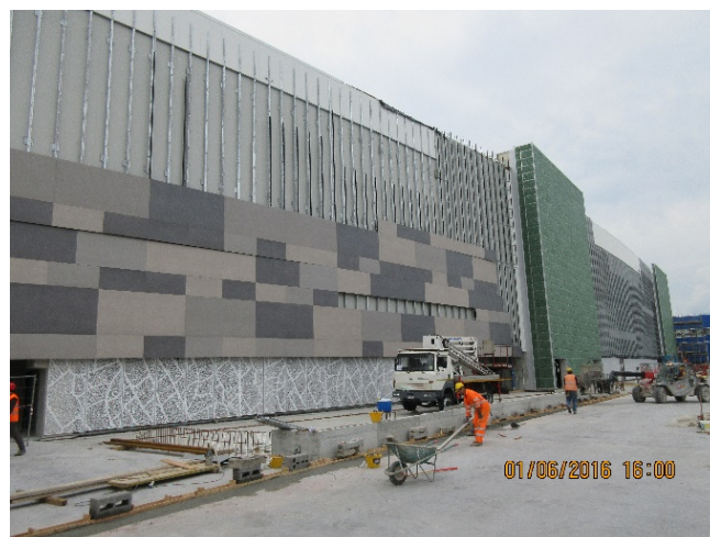
Fig. 3. During Construction (Living wall), Shopping Center, El Nos Roncadelle, Italy (source: authors)
