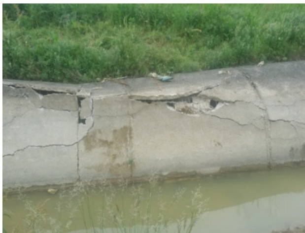
Fig. 9, Current status of a partially restored canal
