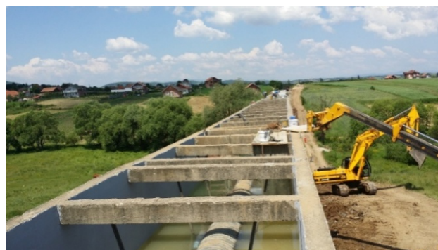
Fig.10, Current status of a partially restored canal
