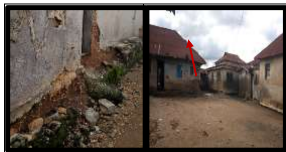
Fig. 3: Typical buildings with eroded foundation and rustic roofs
