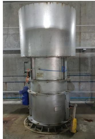
Figure 1: Capture chamber for an OWCs in Mutriku MOWC
