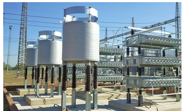
Fig. 26: Shunt capacitors used in distribution grid for reactive power compensation
