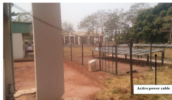
Fig. 22. Solar power Station.
