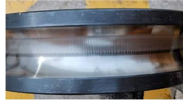
(b) Inner ring failure
