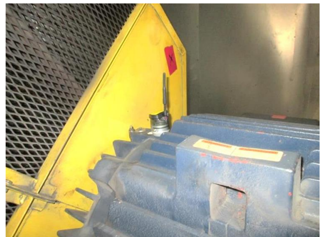
Fig. 7: Vibration Sensors for PdM system
