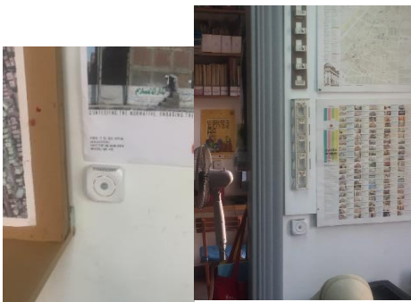
Fig4: Samples of the sensors installed
